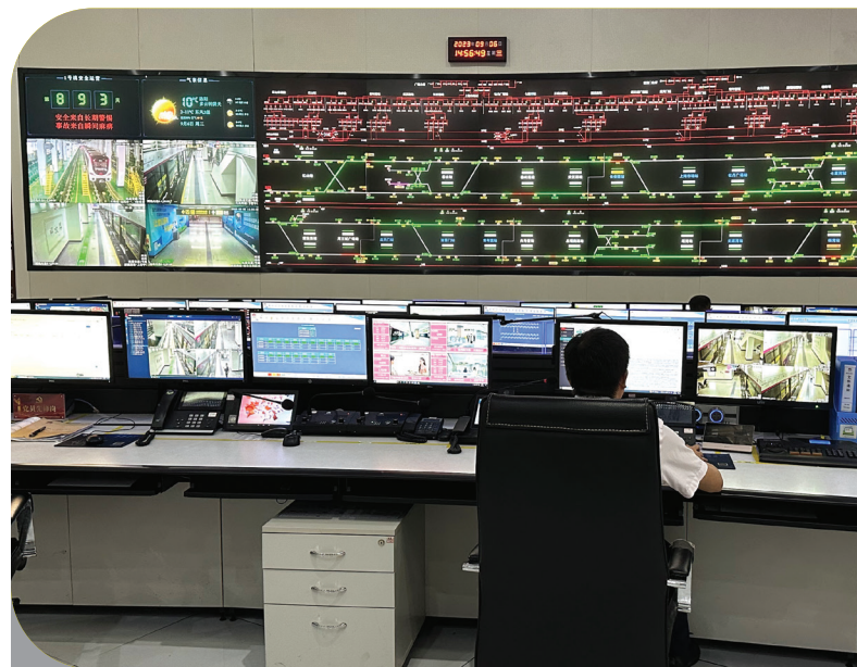
Luoyang Metro Dispatch Control Center
